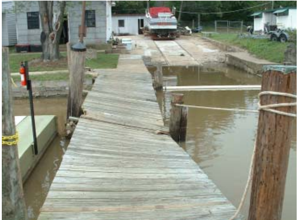
Dock Damage at District Yacht Club
